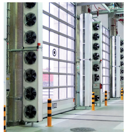
Max Modular towers on large industrial doors
